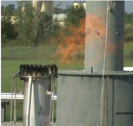
Flare DRE 99.2% at steam-to-vent gas (SVG) ratio of 0.29.
